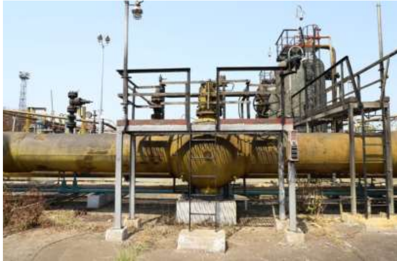
(f). Open FLP fitting (probable ignition source)
