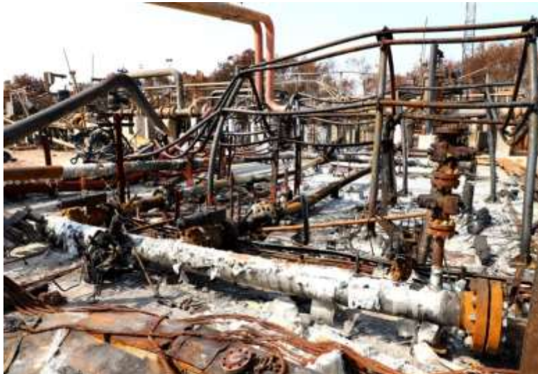
(c). Damaged pipelines
