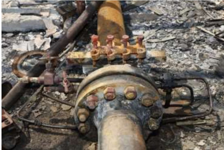
(b). Plate of meter 310FT02 in place
