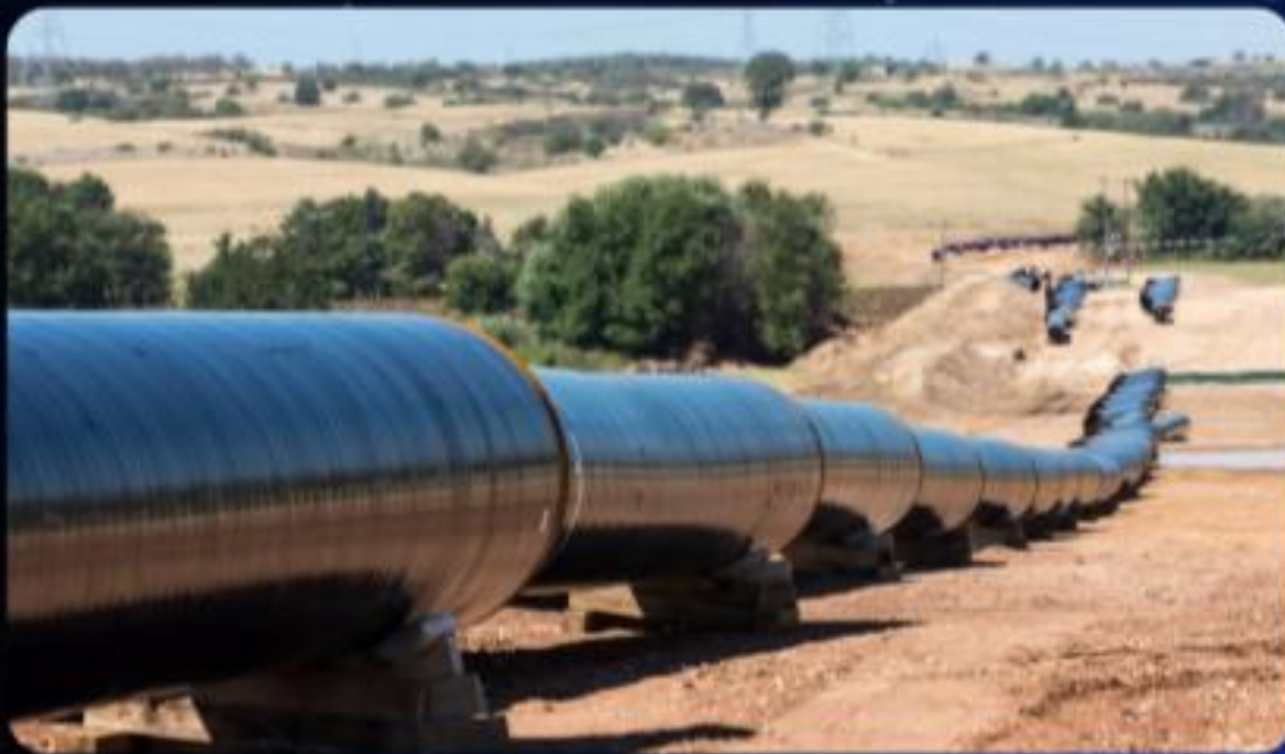
NATURAL GAS PIPELINE (NGPL)
