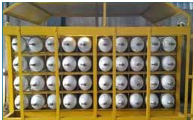
Typical CNG cascade
