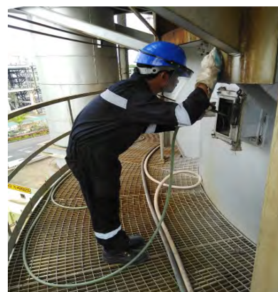
Chemical injection into DHDS heater
