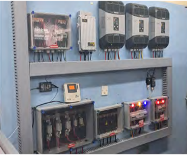
Hybrid Inverter, Charge controller & Protections
