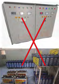
Lead-acid Battery Bank
