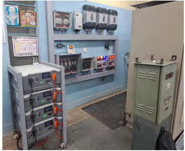
Lithium Iron phosphate (Lifepo4) Batteries
